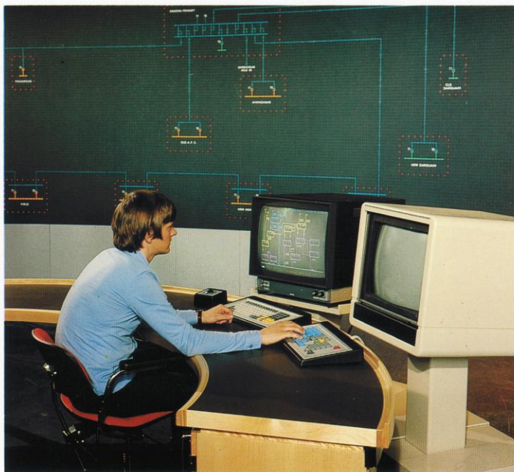
Fig. 7. Control rooms are one of ASEA's specialities. The operator is considered the central figure and around him is built up the ergonomically designed control room interior which also includes the computer software. The illustration shows, amongst other things, ASEA's portable low-profile keyboard. The example on the right shows that diagrams can also be created directly from the keyboard.
