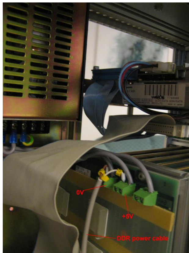
Figure 12 The 0V and +5V power screw terminals in the MasterView cabinet.
